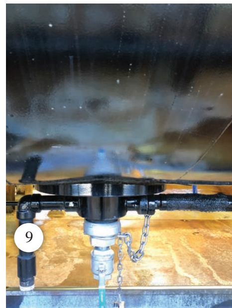
Steam Coil Connection; Top Operated Bottom Outlet Valve and 2" Auxiliary Valve
