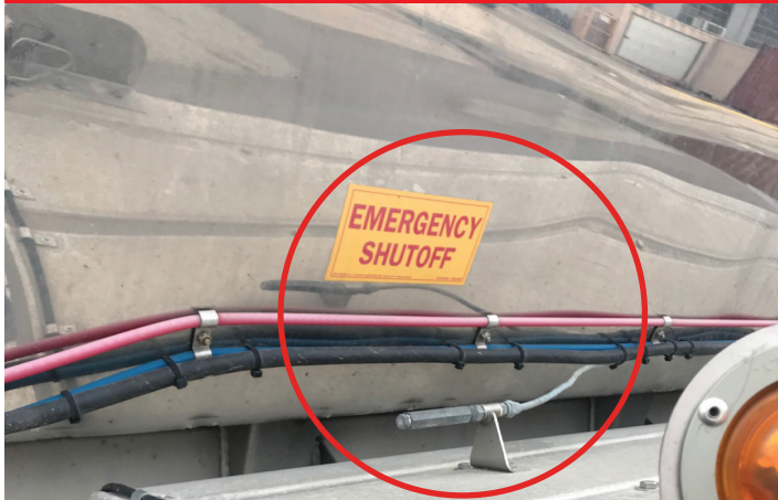
Figure 8: Typical Emergency Shut-Off Device
